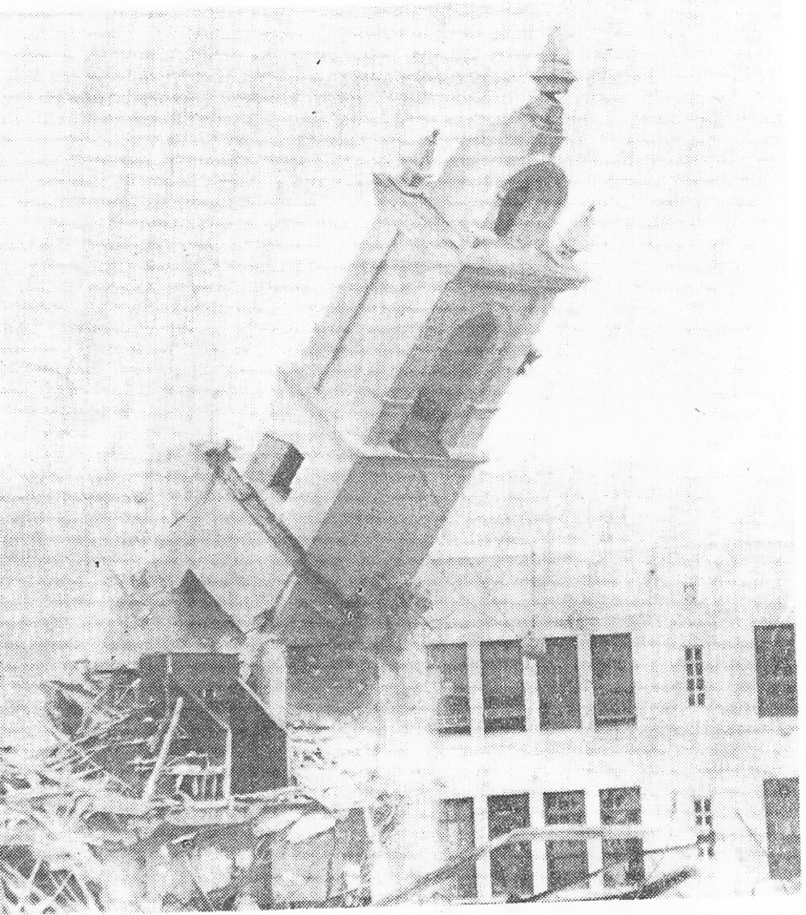
END OF ERA—A landmark which has been standing at 21st Street and Broadway for the past 41 years fell under the “headache ball” of a construction crew today. The bell tower of the Christian Brothers School was brought down to clear the area for the construction of a new Roman Catholic girls high school. Bee Photo by George Roberts
