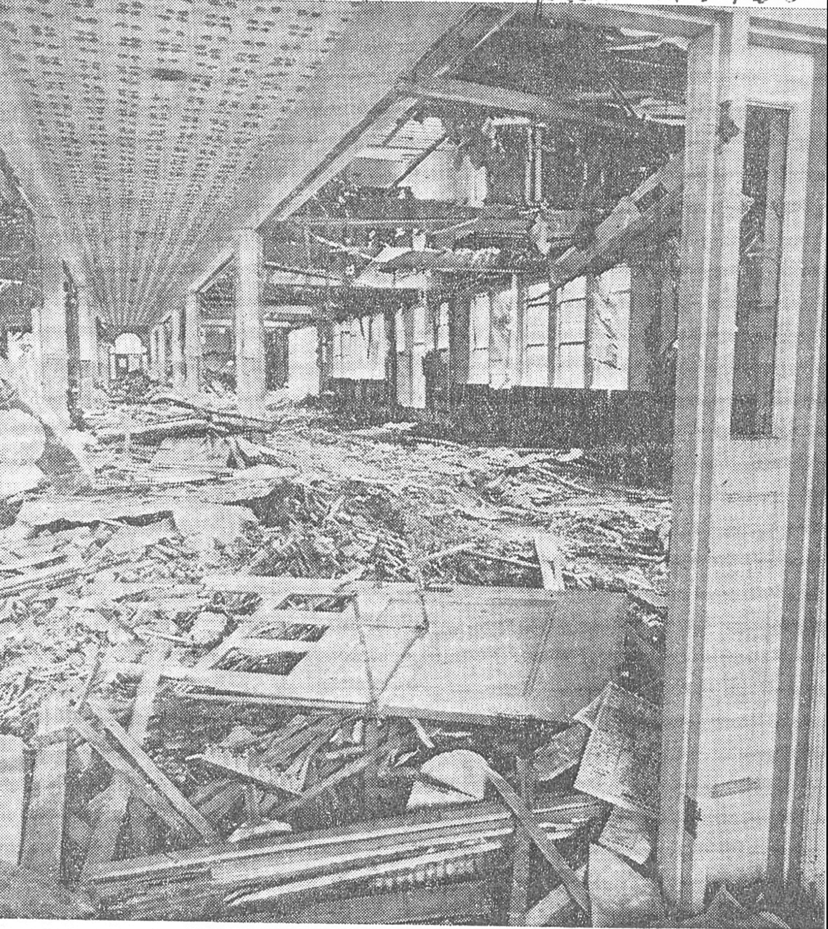
THE THREE R'S . . . Reading, 'riting . . . now rubble. The Christian Brothers school at 21st and Broadway is quickly being reduced to rubble under the onslaught of the wrecker's iron ball. The famed education plant, built in 1924, will be replaced by the St. Joseph's Girls High School.
