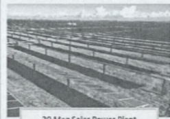
30 Meg Solar Power Plant
