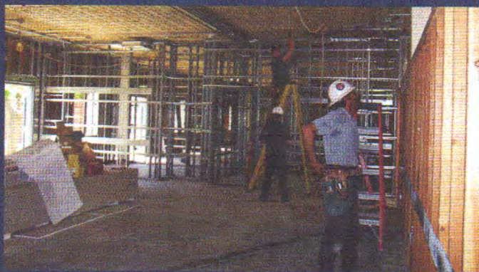
Above, construction crews are remodeling the east annex building into new choir, music and science classrooms. Renovation began in the spring and will be completed before the start of the 2006-07 school year.
