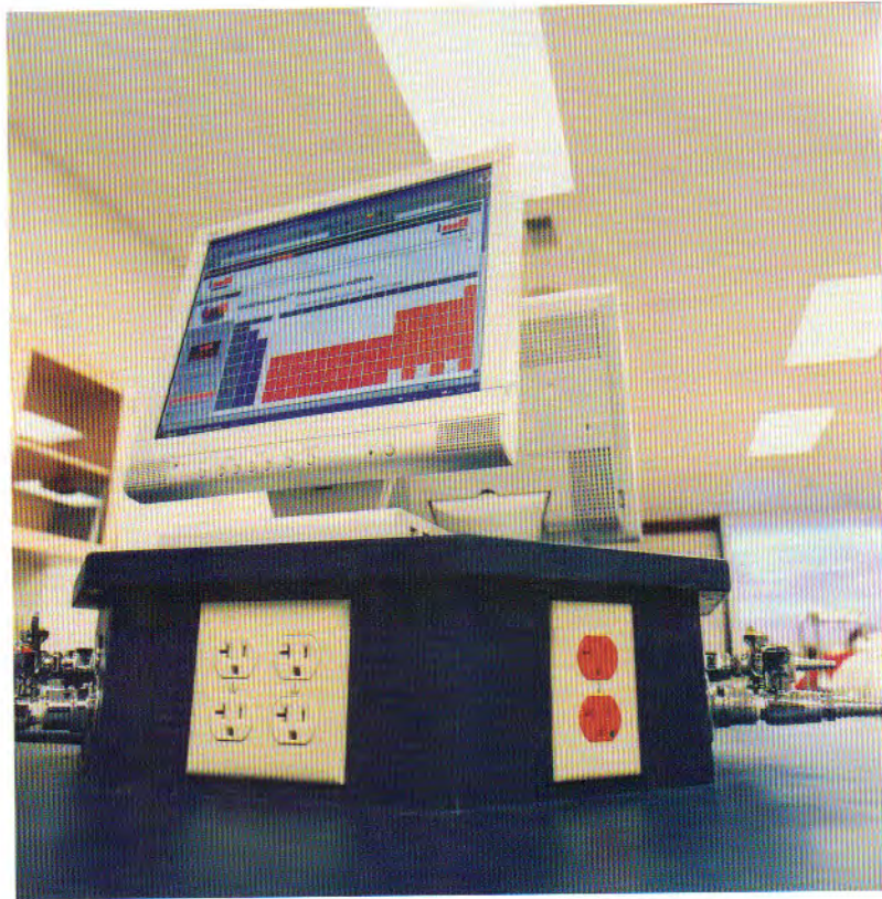
There are thirty-seven separate electric circuits.
