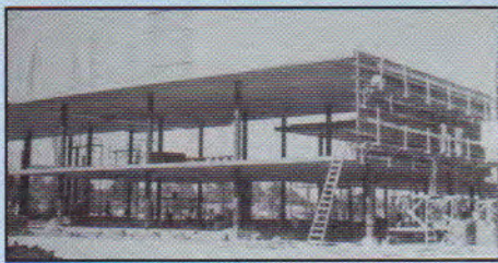
MARCH 1956 → Construction of new school began at the Sacramento Boulevard site (now Martin Luther King, Jr. Boulevard).
